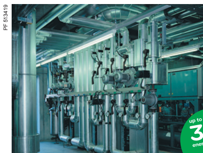
ATV12 controlling a pumping station
