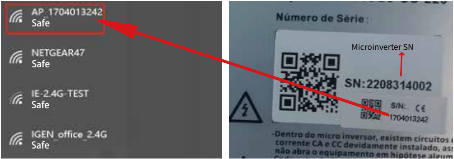
Microinverter SN: 2208314002 Built-in datalogger :1704013242
