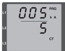
Fig. Current transformer programming mode Use button 1 and 2 to change primary and secondary current (see page 50).
