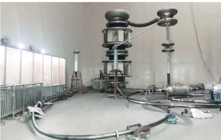
High voltage test
